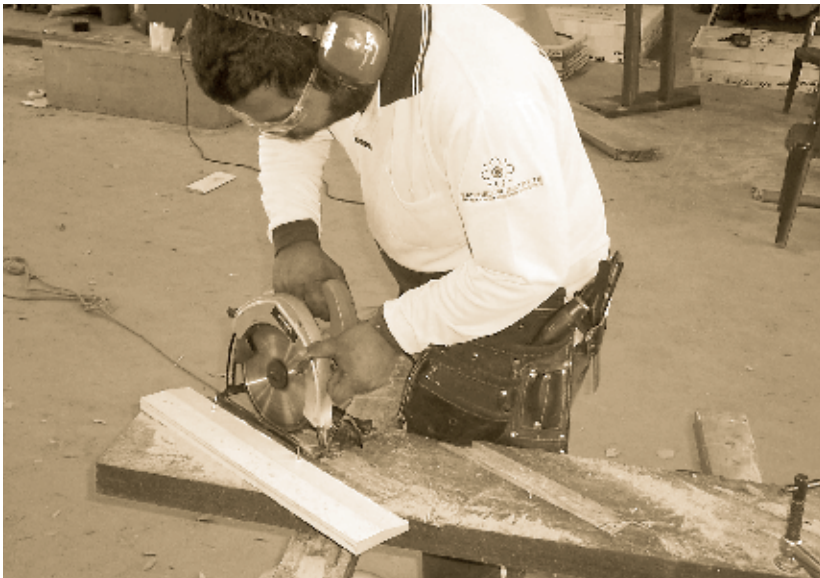
Apprentice Alex MacIntosh working on a set of stairs for the Boggabilla/Toomelah Project.
