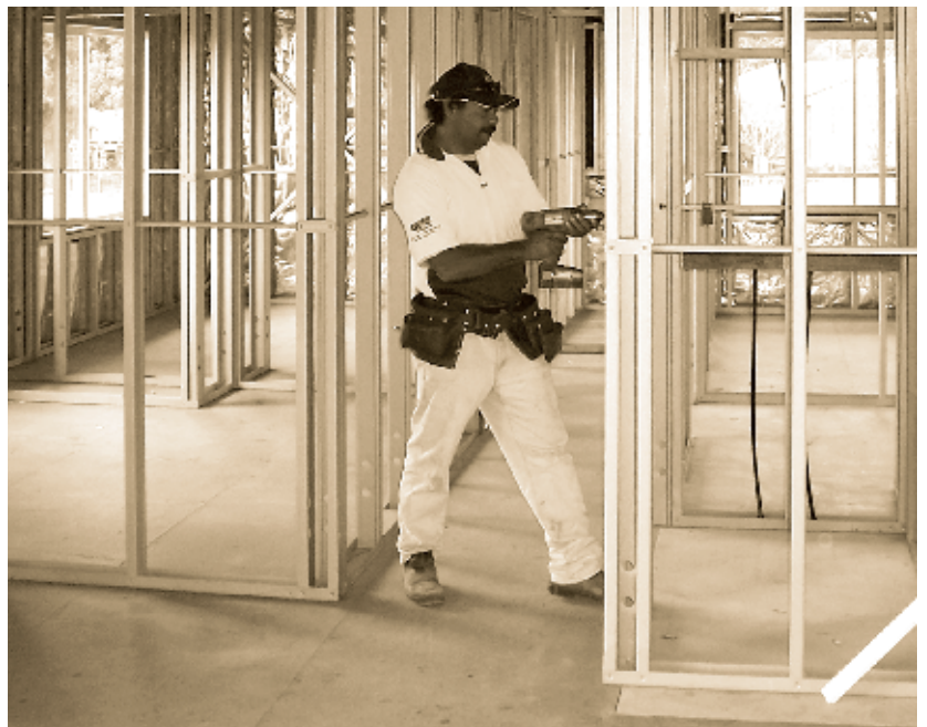
Apprentice Reginald McGrady working inside the "apprentices' house" on the Stage 3 Boggabilla/Toomelah Project.
