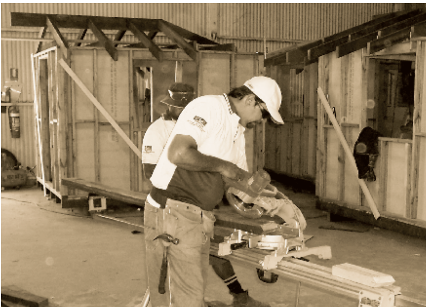
Arnold McGrady cutting angles for the roof construction on the Boggabilla/Toomelah Project.
