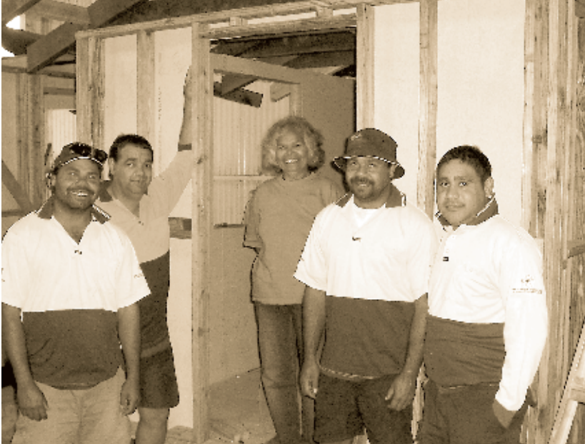
Mike McGrady, Lonnie Duncan, Elaine Edwards, Reginald (Dickie) McGrady and "PJ" Duncan with timber storage sheds on site at the Toomelah and Boggabilla housing and infrastructure project.
